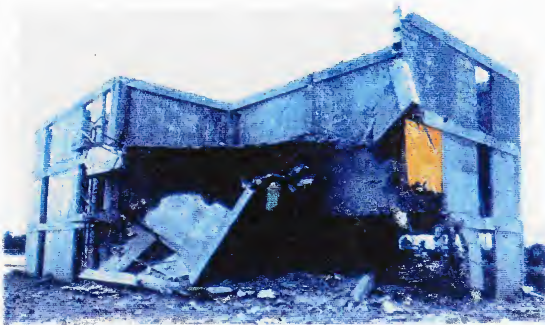
Figure 3. Damage Resulting from Internal Detonation of 180 lb TNT Equivalent
