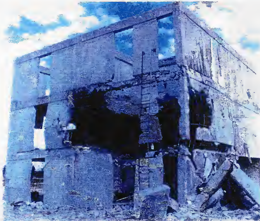
Figure 4. Damage Resulting from Internal Detonation of 35 lb TNT Equivalent
